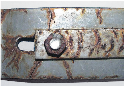
Fig. 8: SCC of a bracket made of the material 1.4301 (A2, 304) after approx. 4 years of use in an indoor swimming pool.
