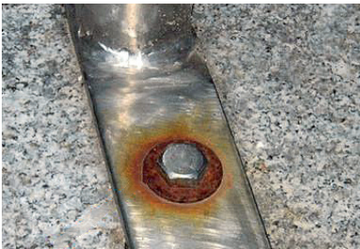
Fig. 12: This is a typical case of contact corrosion. Zinc-plated carbon steel (washer) and stainless steel (screw and part) were used together. The surface area of the more noble metal – the stainless steel – is larger, causing heavy corrosion of the washer.
